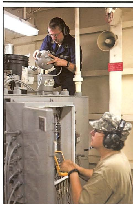
Chief Warrant Officer Vicky Lipps, the first engineer (bottom right), and the Chief Engineer John T. Owens II both with the 548th Transportation Detachment struggle to fix a power glitch in the Kuroda's hydraulic wench anchor system in the bow thruster room of the ship. (Top) Owens changes filters that were melted by hydraulic fluid.
